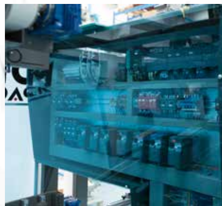
Electric cabinet on view for an immediate diagnosis.
